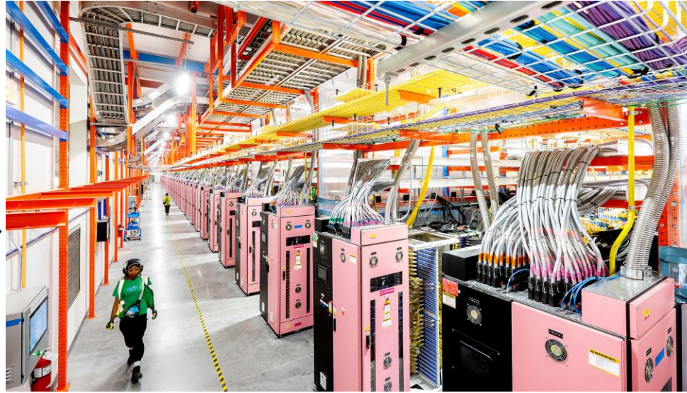
Several accelerator-equipped servers are connected to form a single, datacenter-scale inference and training fabric.
